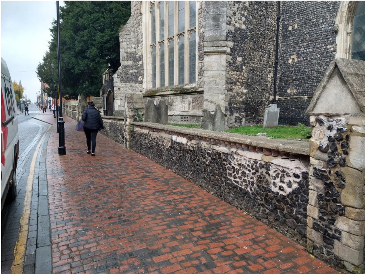
High Street public realm and boundary to St Michael's Church in need of repair
